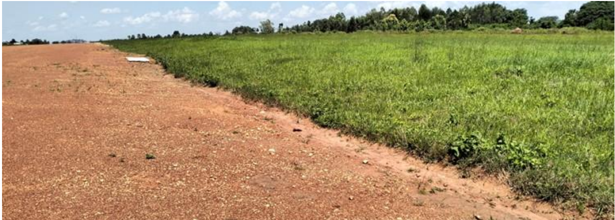
Figure 6: Some of the most evident scoring of the runway due to rampant erosion due to drainage challenges at the Aerodrome
