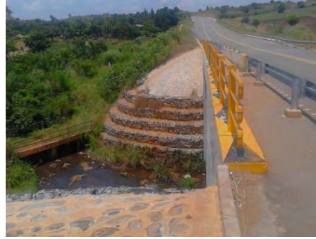
State of flow at Rutoha Bridge along Hoima - Kaiso/Tonya Road. The flow is too low for a river intake, an impounding reservoir would be required.
