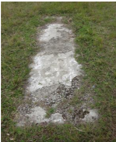
Figure 25: Runway markers broken, fade, overgrown
