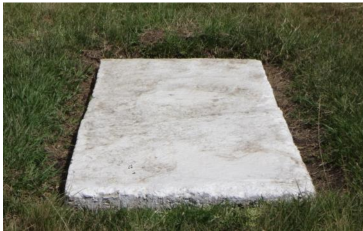
Figure 26: markers surrounded by a gap, not flush with the runway surface or dealthalised
